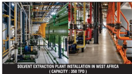
SUNFLOWER OIL EXTRACTION PLANT INSTALLED IN WEST AFRICA (CAPACITY : 250 TPD)
